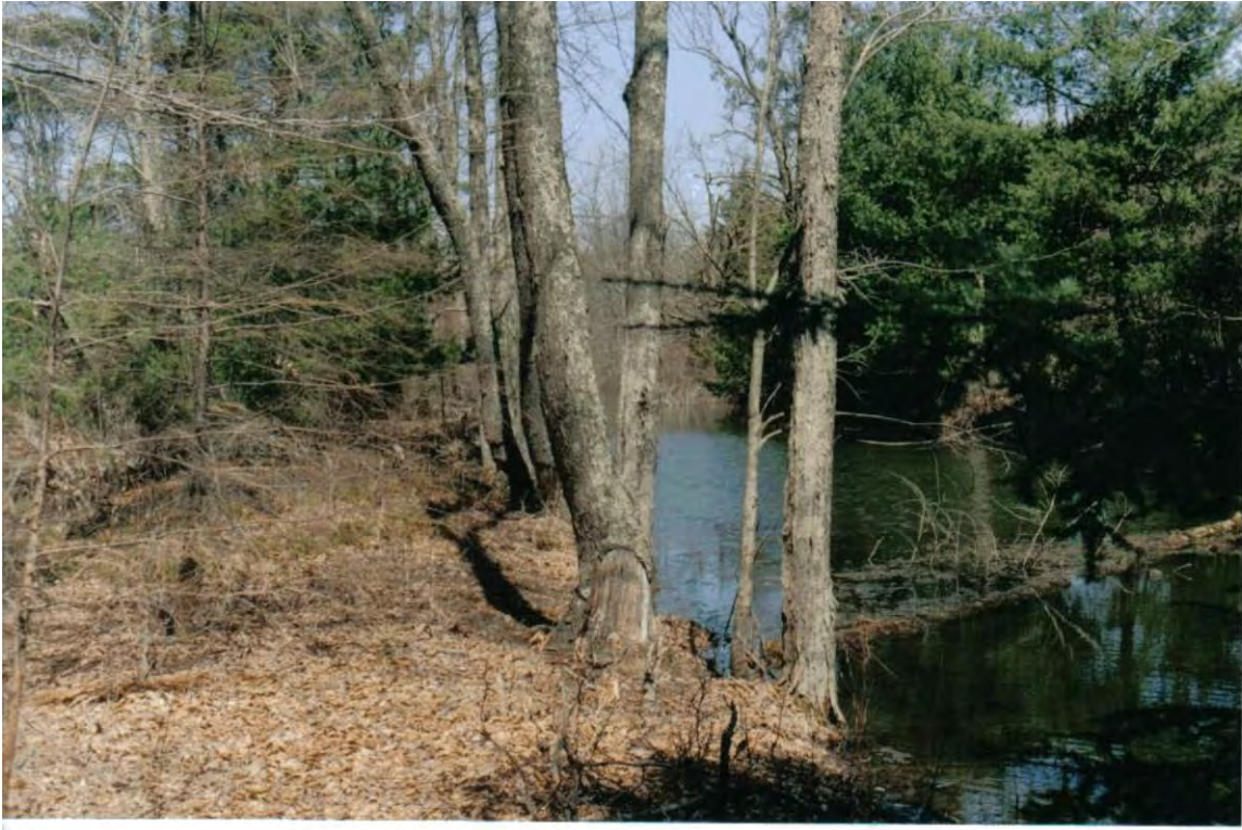
Looking north along the tow path into Chenango County. Trees and brush are growing on the tow path. Water fills the prism.
