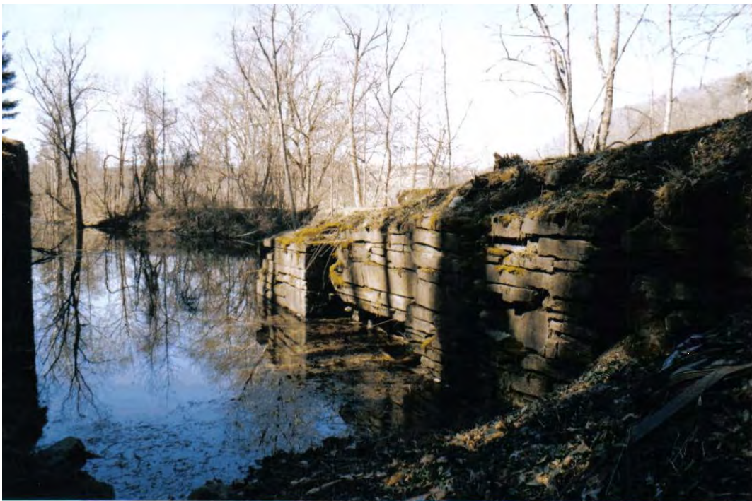
Above - east wall. Below - west wall at the south end of the lock
